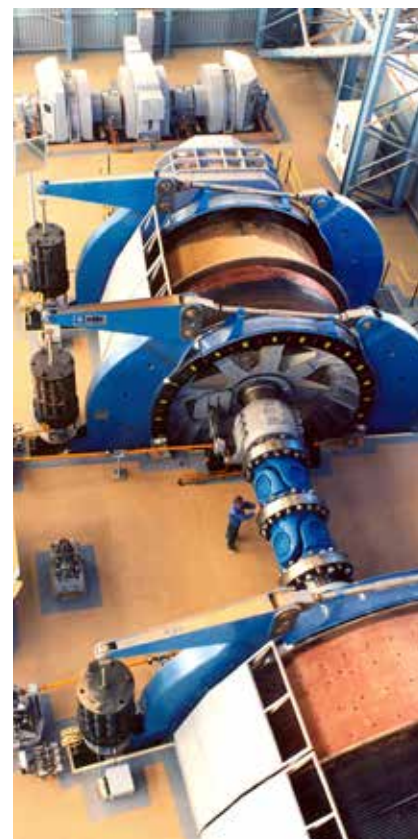
Ø 5.1m BMR Hoist with Hookes Joint Coupling - South Deep
