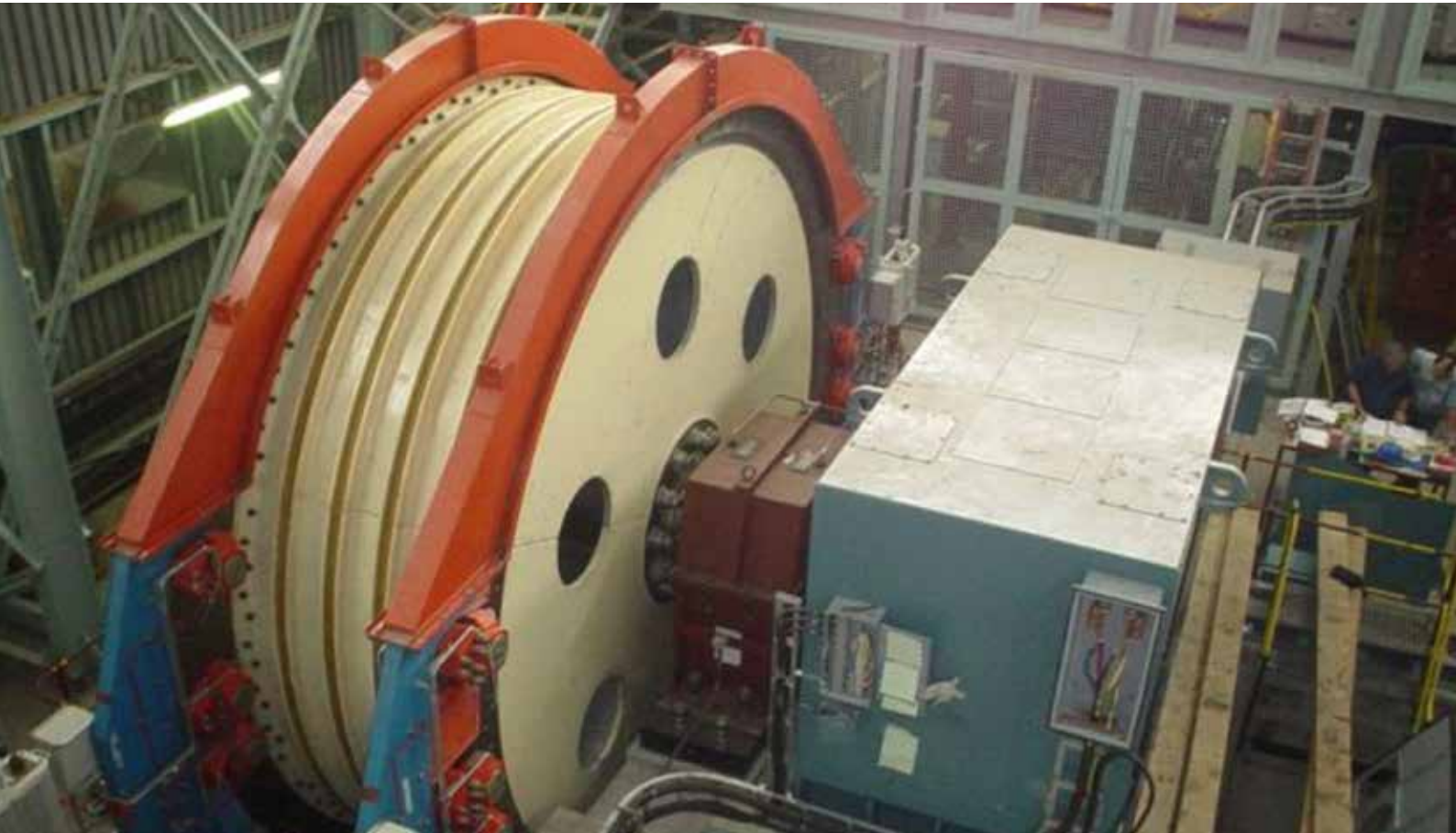
Ø 6.0 m 4-Rope Koepe Hoist - Lonmin K4.
